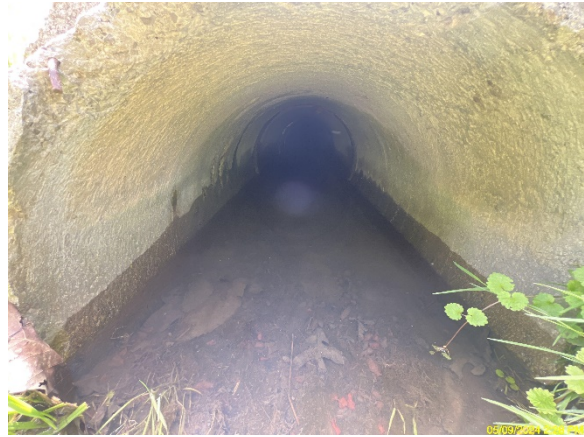
Figure 22: Pipe blocked less than 25%.
