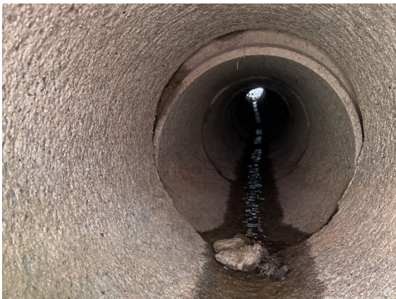
Figure 3: Concrete pipe with abrasion and minor misalignment of pipe sections.
