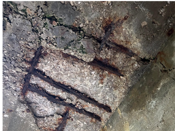
Figure 14: Concrete box culvert with localized spalling and corroded reinforcing steel.
