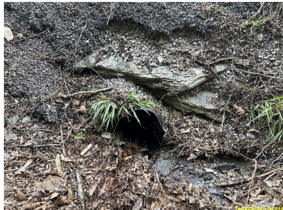
Figure 6: Distorted HDPE pipe end with some damage.
