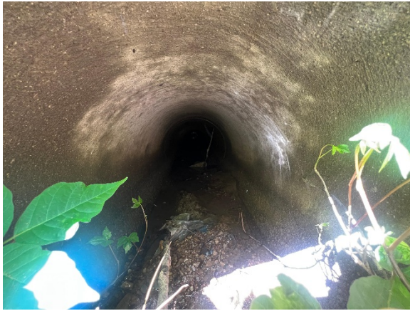
Figure 21: Pipe blocked less than 25%.
