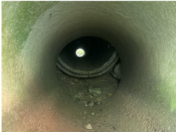
Figure 9: Significant pipe section misalignment.
