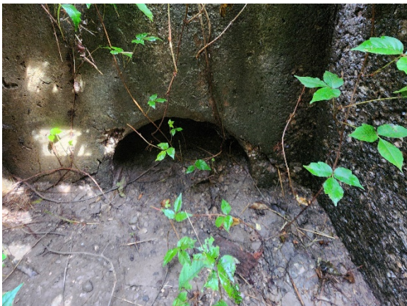
Figure 25: Pipe up to 50% blocked and functionally inadequate.
