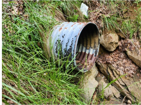
Figure 2: Steel pipe with insignificant corrosion.
