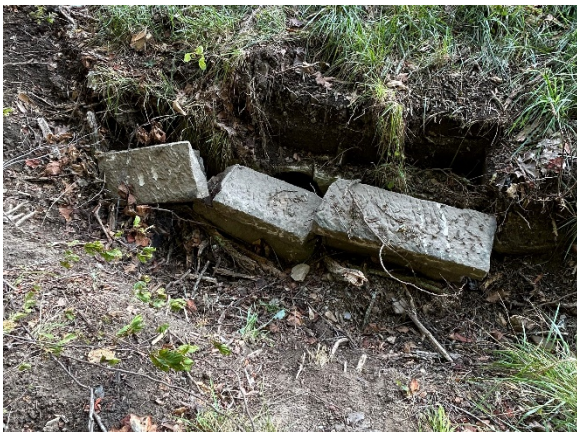
Figure 15: Failed headwall and collapsed pipe end.
