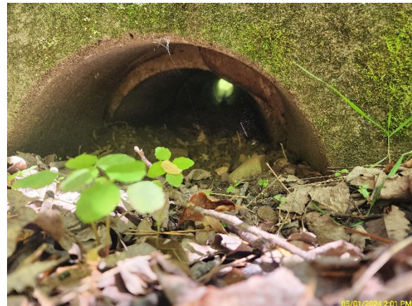
Figure 24: Pipe 50% blocked and functionally inadequate.
