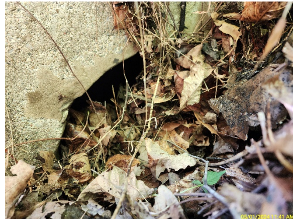
Figure 30: Pipe greater than 50% blocked and functionally inadequate.
