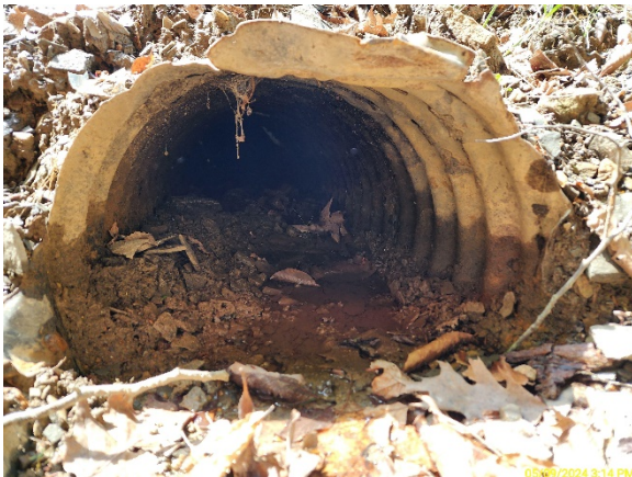
Figure 23: Pipe 25% to 50% blocked and functionally inadequate.
