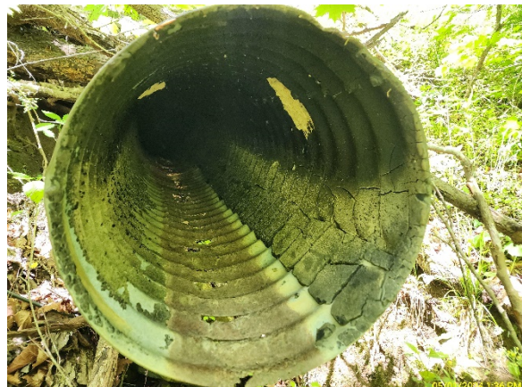
Figure 4: Steel pipe with minor corrosion and perforations forming.
