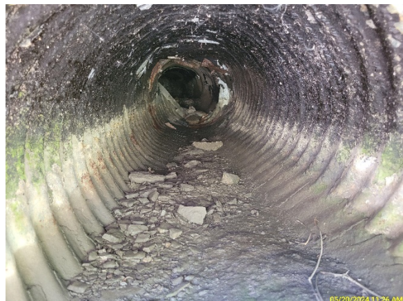
Figure 12: Pipe separation and significant corrosion.
