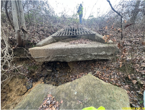
Figure 7: Significant scour away from roadway with separation of apron from end section.
