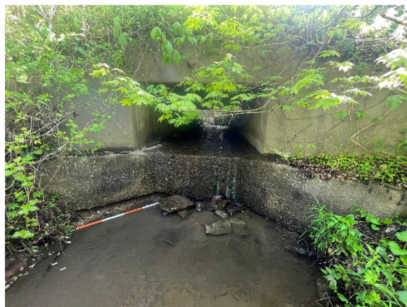
Figure 5: Concrete culvert with minor scour and abrasion at curtain wall and bottom slab.
