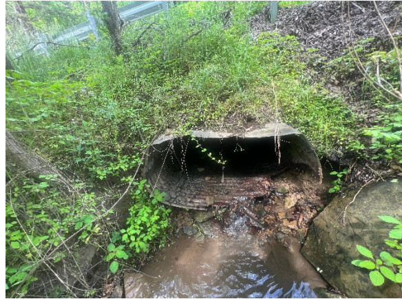
Figure 8: Significant distortion of pipe with large perforations.
