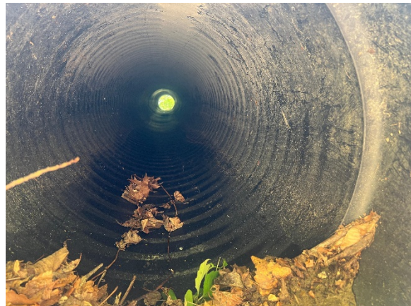
Figure 20: Pipe less than 10% blocked and functionally adequate
