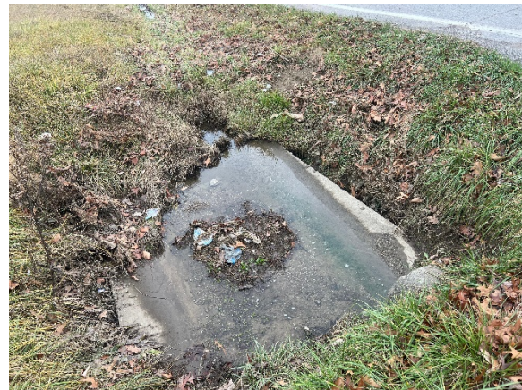
Figure 32: Pipe 100% blocked and non-functioning.
