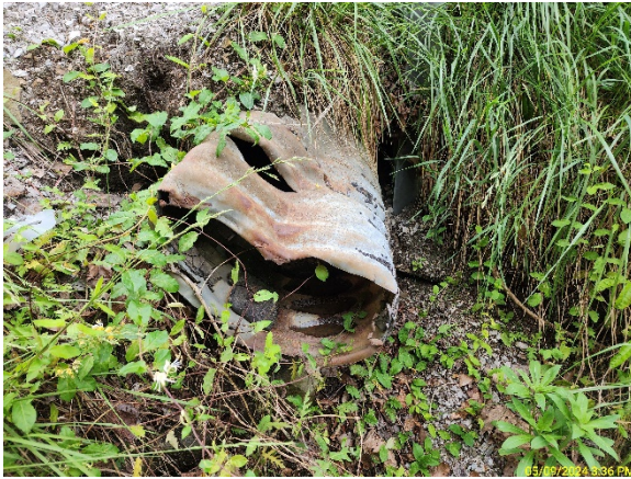
Figure 27: Pipe collapsed and functionally inadequate.
