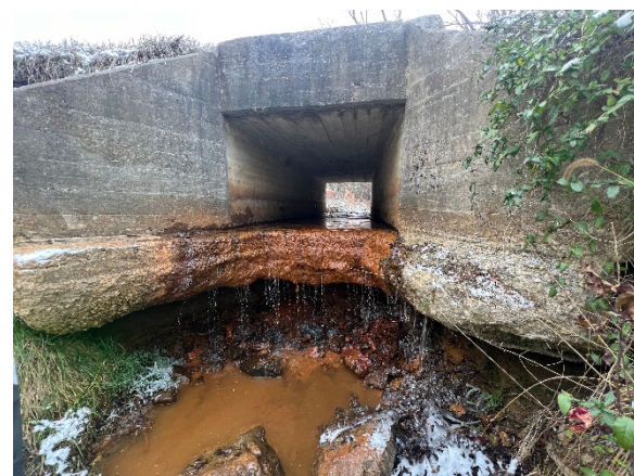
Figure 17: Heavy scour of bottom slab and wingwalls encroaching below roadway
