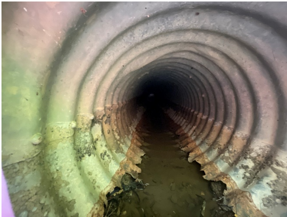
Figure 13: 18" diameter steel pipe with significant corrosion.
