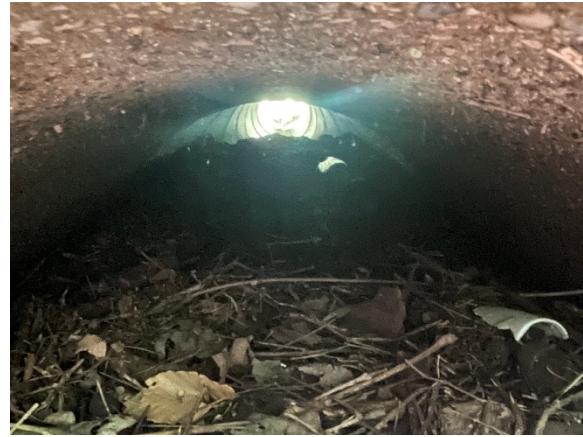
Figure 28: Pipe greater than 50% blocked and functionally inadequate.
