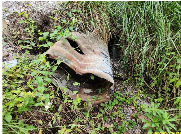
Figure 10: Crushed pipe end.
