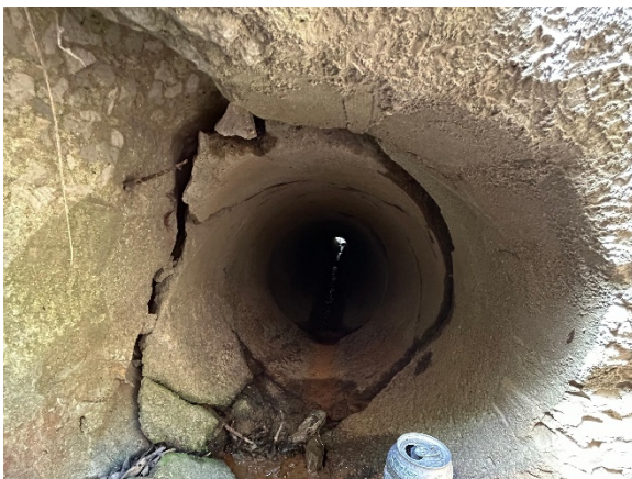
Figure 11: Crushed pipe section.
