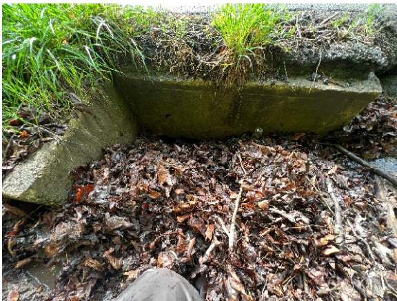
Figure 31: Pipe 100% blocked and not functioning. Pipe 100% blocked and not functioning.
