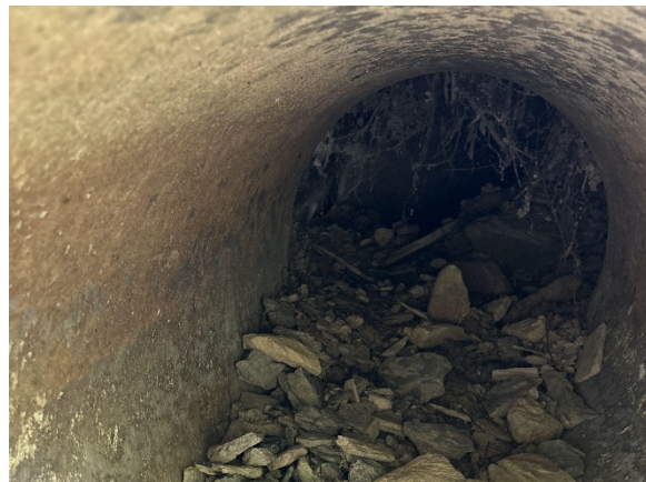
Figure 26: Pipe 25% to 50% blocked and functionally inadequate.
