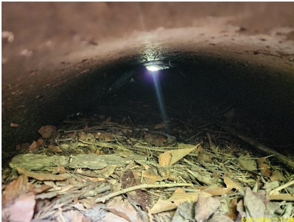
Figure 29: Pipe greater than 50% blocked and functionally inadequate.
